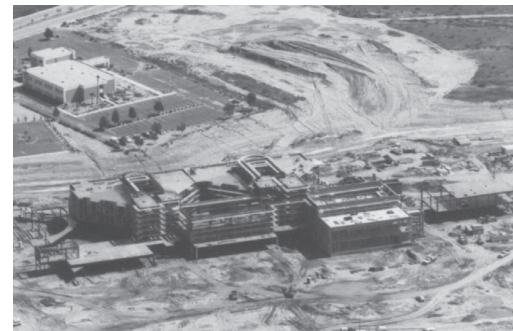
Shea Medical Center, under construction in this aerial photo, was made possible by community support and Scottsdale Healthcare Foundation.
